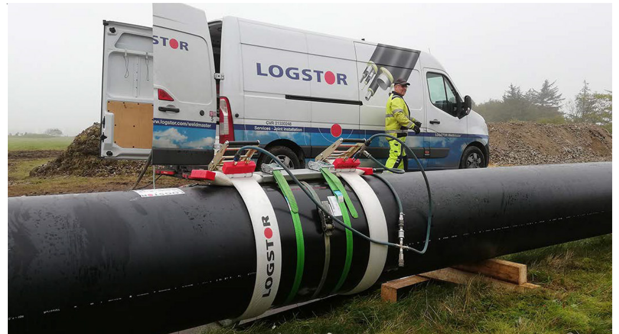
Complete set of pressing tools and LOGSTOR WeldMaster/ WeldMaster Light. The welding pressure is maintained with air pressure which is continuously checked during installation.
